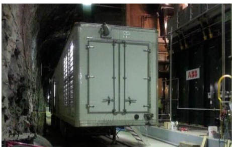
EOK-TORS 6000 at underground generating station
