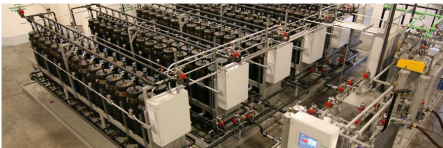
Large Scale Unattended Tank Farm Operation
